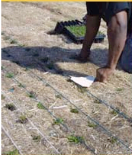
Planting the plugs of sedum through the coconut fiber mat, following the landscape architect's design.
